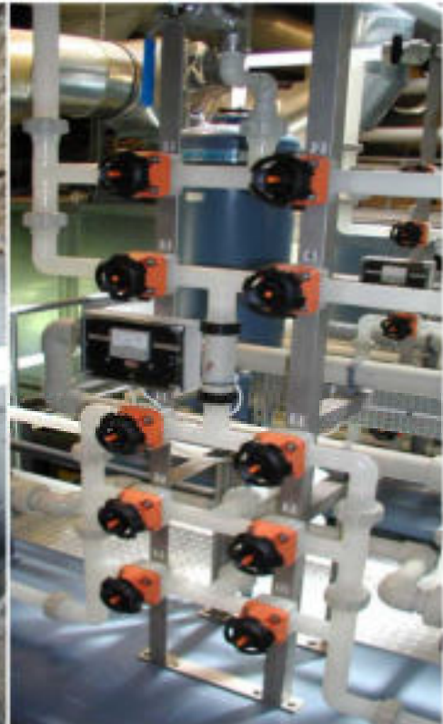
PP-n pipe system used for Mill Q water
